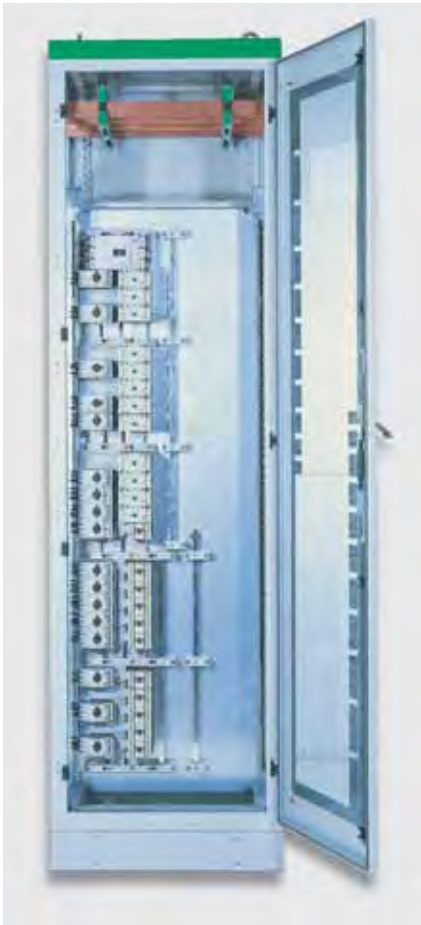
Photo 6: Motor starter section from an engineered product assembly featuring a vertically mounted busbar array to accommodate a large number of motor starters.
