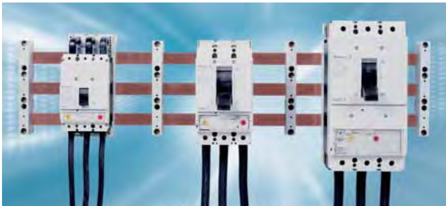
Photo 3: It has become possible in the meantime to design adapters which allow mounting of circuit breakers or molded case switches, rated up to 550 A and used in incoming or outgoing circuits, directly onto the busbar system. The actuation possibilities for the switches can also be varied, from manual means to remote switching via an electrical motor operator, or even through a flex cable and side handle accessory typical of North American installations.
